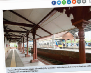
The station is in a state of disrepair and needs a major overhaul.
