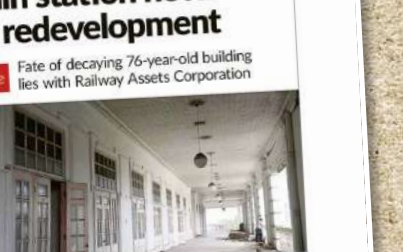
The building is in a state of disrepair and needs a major overhaul.
